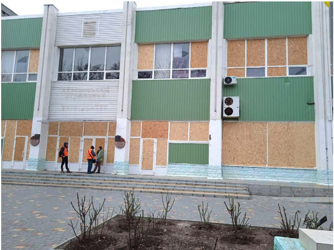
Bombing explosion waves damaged the façade and broke the windows of Kherson State University. After Kherson was deoccupied, the windows were temporarily “glazed” with OSB panels.
