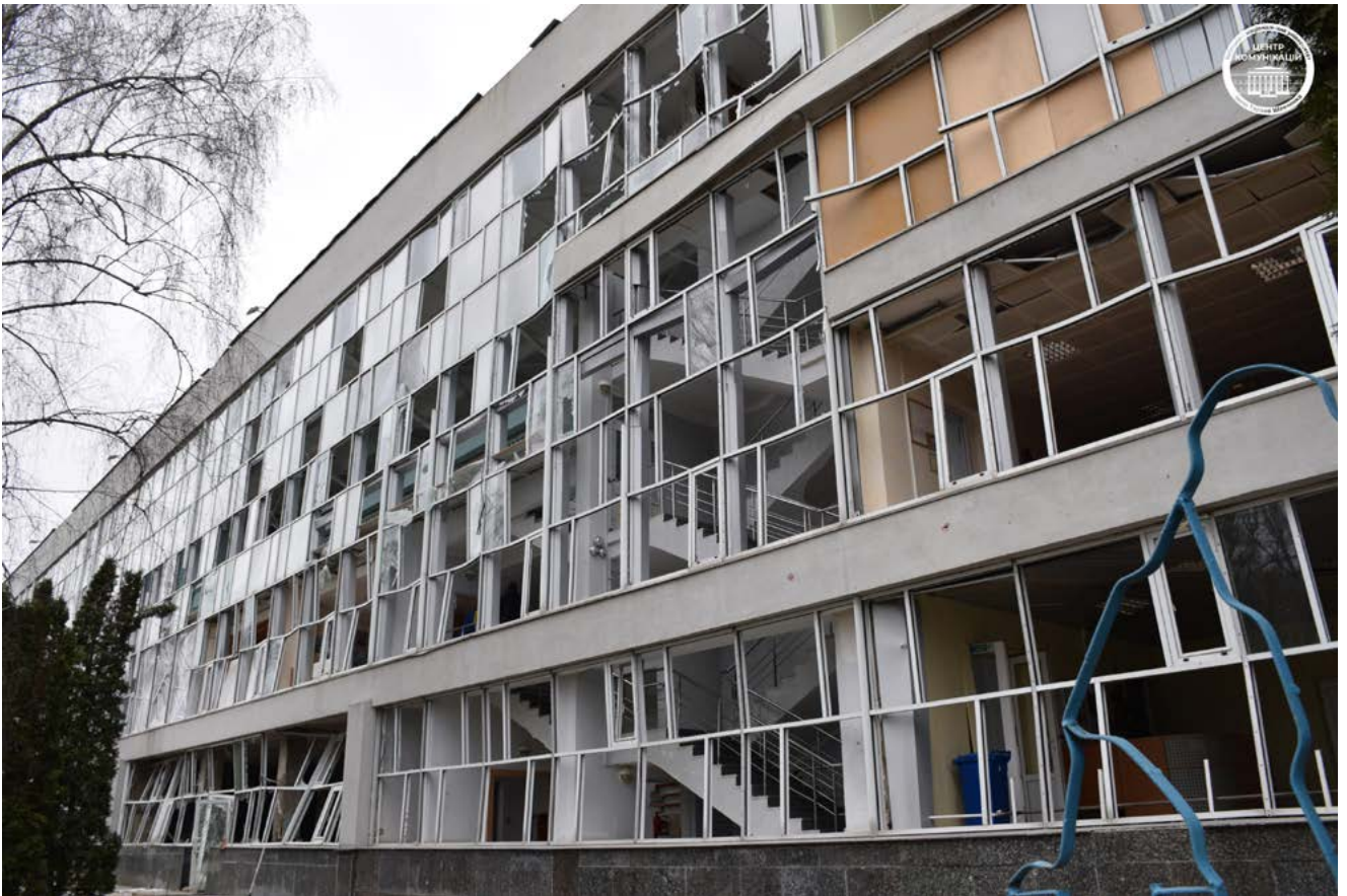
Taras Shevchenko National University of Kyiv buildings damaged by the July 10 and December 31, 2022 shellings.
